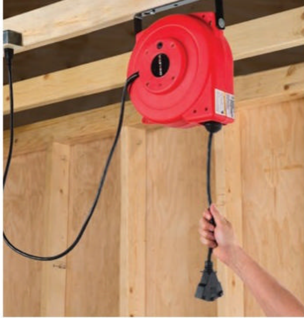
A single ceiling outlet, paired with a retracting extension cord, can easily supply electricity to just about any spot in a small shop
