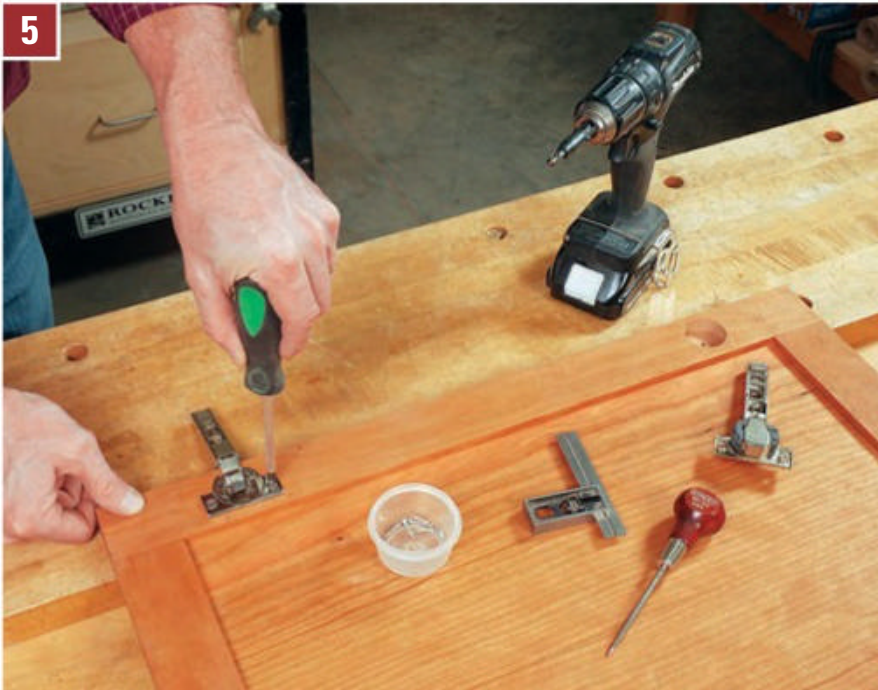
5 Drill pilot holes for the hinge cup screws with a 3/32" self-centering bit. Then drive in the screws to secure the hinge cups in their mortises. Installing these delicate screws by hand will help prevent breaking them.
