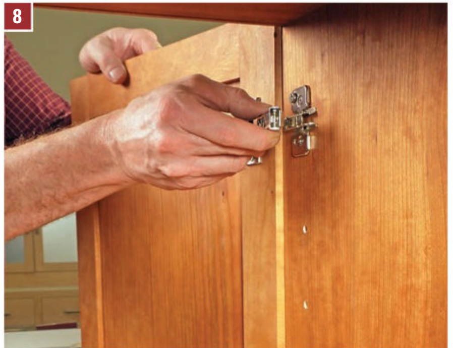
8 Set the door into position on the cabinet, and snap the long-arm portion of the hinges onto the mounting plates to hang the door. (If this were a compact hinge instead, the hardware would be a single component.)
